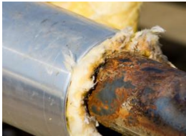
Figure 2: Corrosion under Insulation, Image from North County Mechanical Insulators Website, http://www.ncmiinc.com/corrosion-under-insulation
