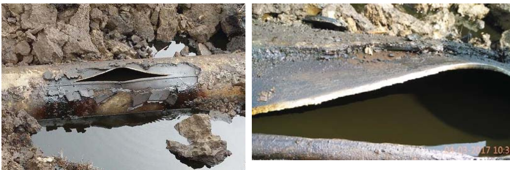
Figure 1.9: Seam failure of Crude Oil Pipeline due to corrosion/ micro cracks in Northern India causing crude oil spillage
