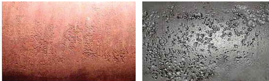
Figure 1.8 Pitting Corrosion on the External Pipeline surface
