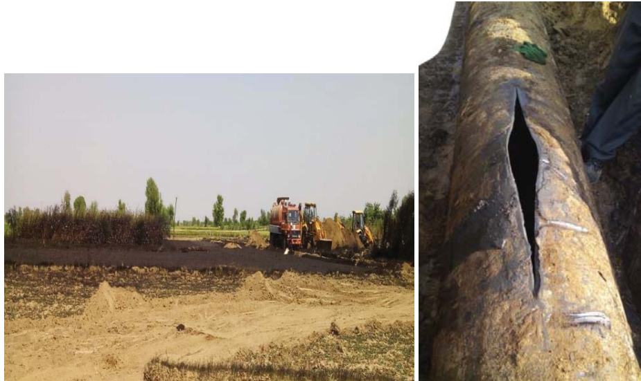
Figure 1.10: Crude Oil Spillage in irrigated field on account of corrosion leakage. Seam opening of pipeline on account of corrosion
