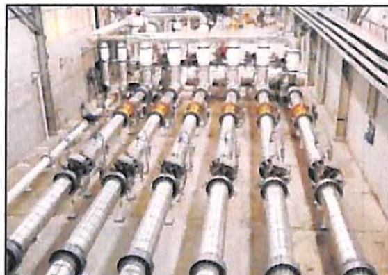
High pressure calibration facility Winnipeg www.instromet.com
