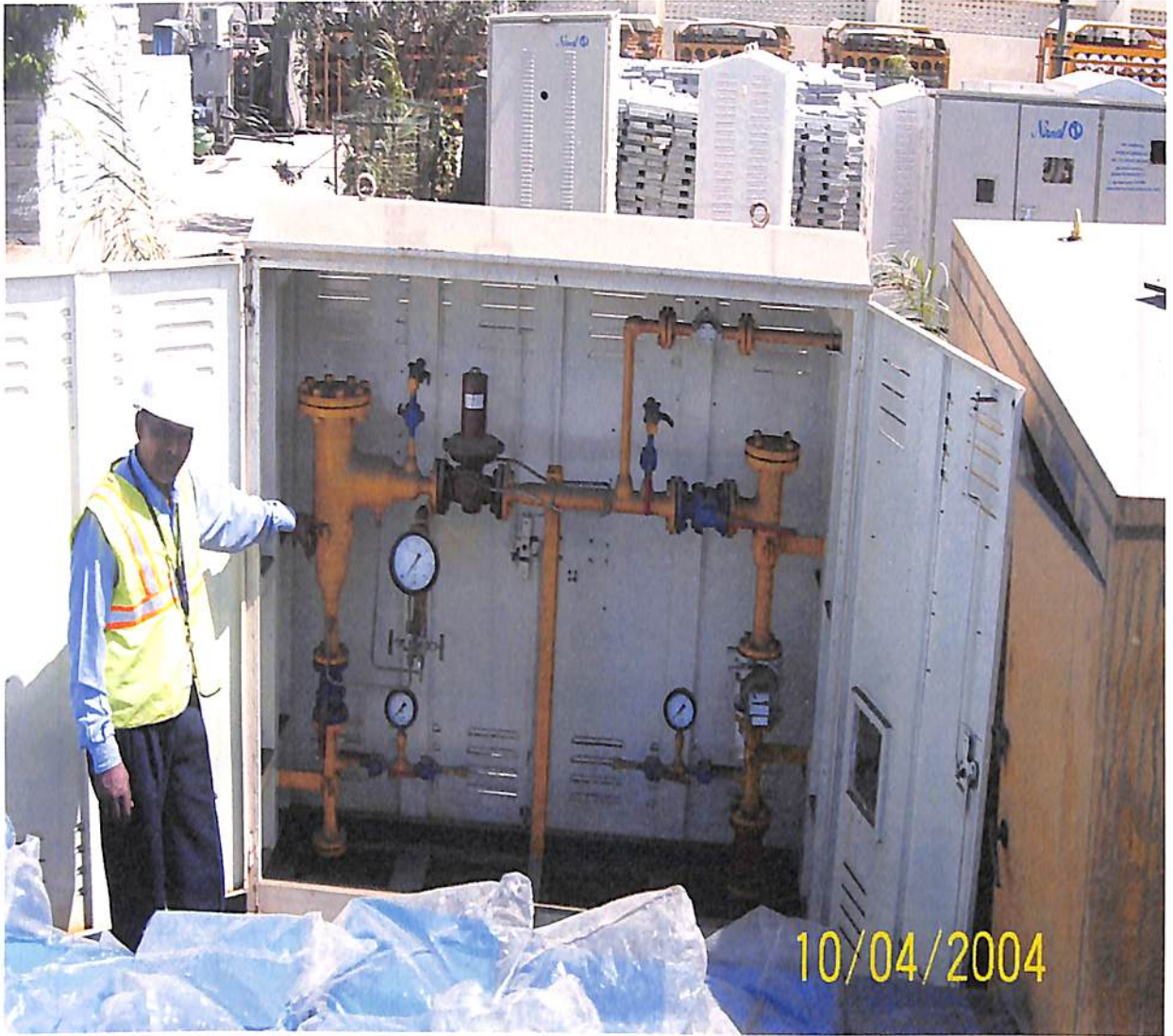
A Metering and Regulating Station (MRS)
