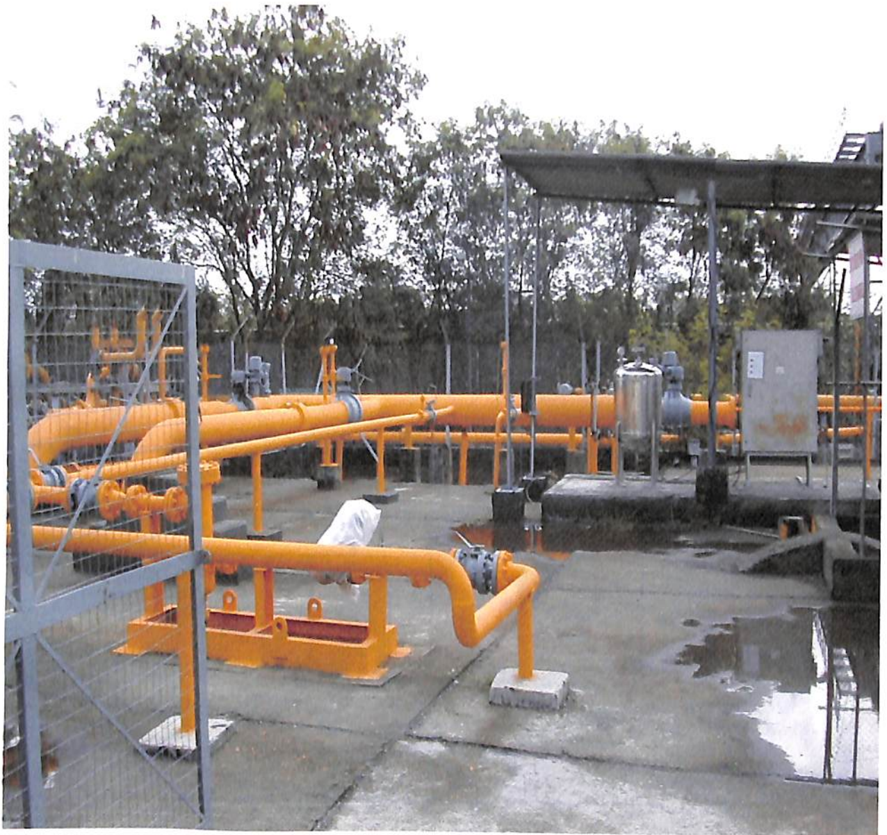
A view of the Gas Terminal at City Gate Station (Mumbai)
