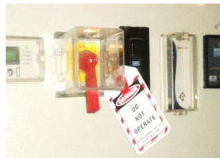
Figure 2-4 Electrical Panel Lockout Device (Make and Image Source -Bradyid)
