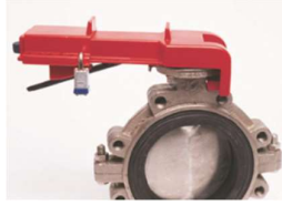
Figure 2-13 Butterfly Valve Lockout (Make and Image Source –E Square)
