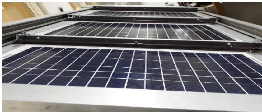
Fig. 5.5 Developed Self-cleaning PV sliding system
