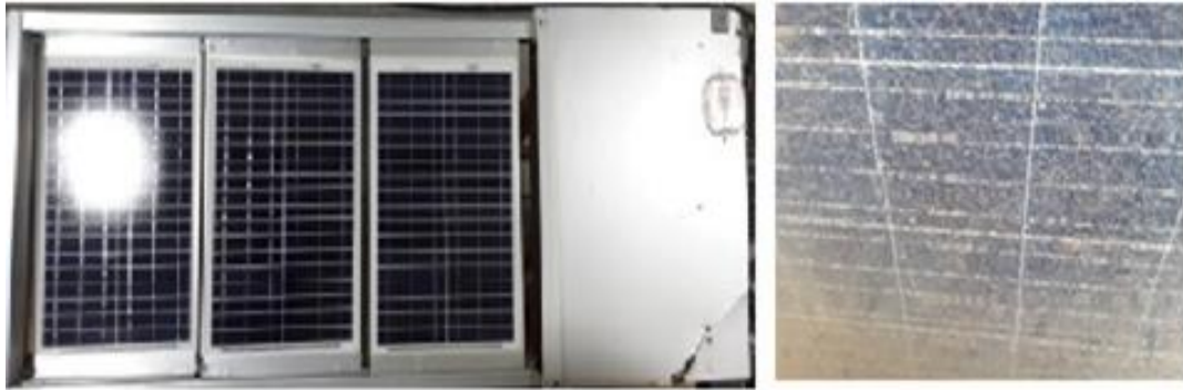
(a) (b) Fig. 5.17 (a). Proposed system after deadly hailstorm, (b) 300W PV panel damaged during deadly hailstorm on 5 March 2020
